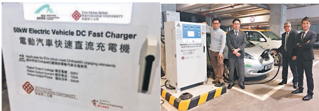
Figure 2: Electric Vehicle DC Fast Charger at the HK Airport Authority (left). Members of UoA12 and representatives from the HK Legislative Council and Airport Authority (right) [Im5].
