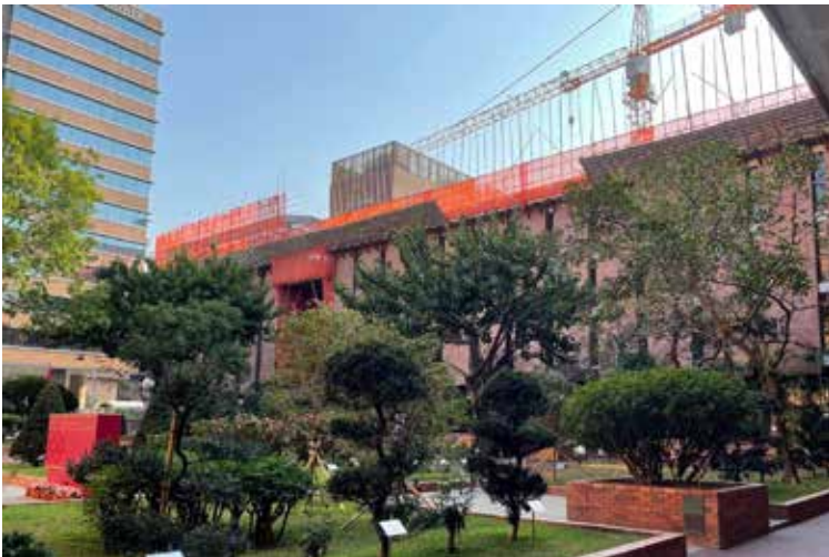
Library Extension and Revitalisation under construction, PolyU 理大施工中的圖書館擴建及翻新工程
