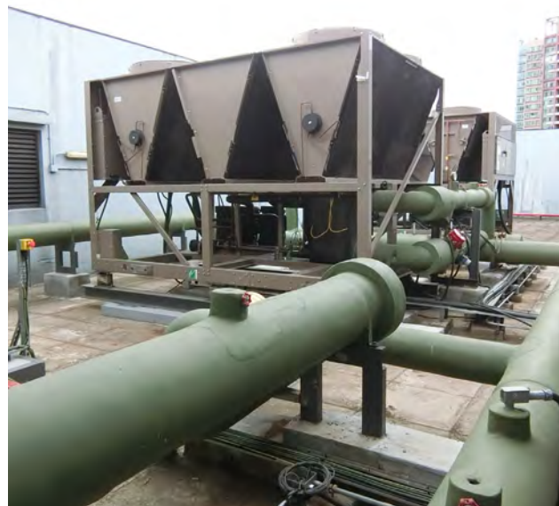
Replacement works of chiller units, chilled water circulation system and building management system for the mechanical ventilation and air conditioning installation, LU 嶺大製冷裝置、冷凍水循環系統及樓宇管理系統更換工程
