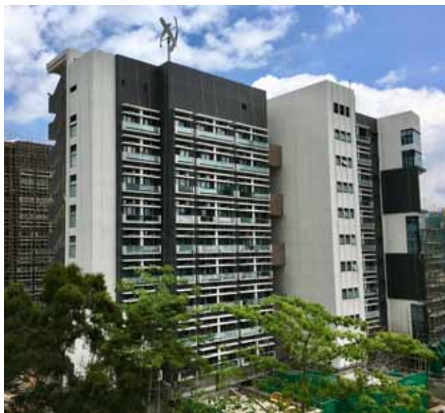
Student hostels on northern campus (blocks A3 and A4) under construction, CUHK 施工中的中大校園北陲學生宿舍 (A3及A4座)
