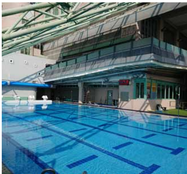
Conversion of the existing swimming pool into an outdoor heated swimming pool at Wai Hang Sports Centre, HKBU 浸大偉衡體育中心戶外溫水泳池改建工程
