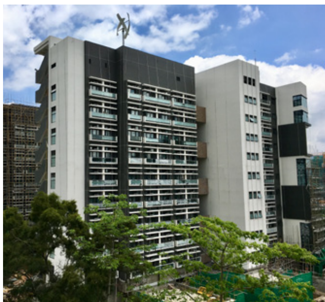
Student hostels on northern campus (blocks A3 and A4) under construction, CUHK 施工中的中大校園北陲學生宿舍 (A3及A4座)
