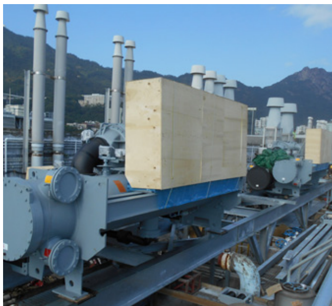
Replacement of air-cooled chillers by water-cooled chillers, CityU 城大以水冷式製冷機替代氣冷式製冷機工程
