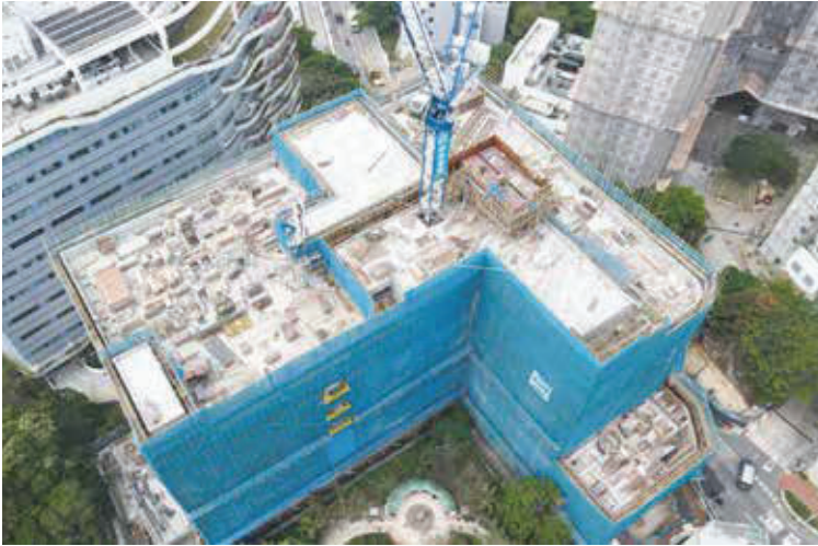
Academic Building at No. 3 Sassoon Road under construction, HKU 港大施工中的沙宣道 3 號教學大樓
